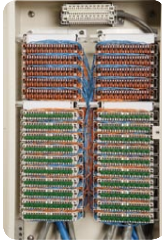
Green activation plugs in cross-connect distribution field provide visual indication of active xDSL customers.
